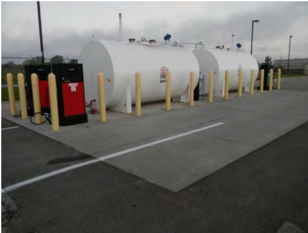
Photograph No 1 AST fueling system at Operations Facility. Tanks are double-walled and fuel sumps are located beneath the dispensers.
